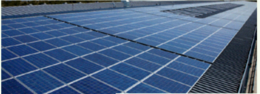
ROOF TOP SOLAR POWER SYSTEM
